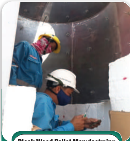
Black Wood Pellet Manufacturing Plant Project in Binh Dinh
