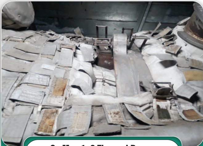
Ca Mau 1, 2 Thermal Power Plant Project
