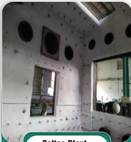
Soltec Plant - Nhon Trach Project
